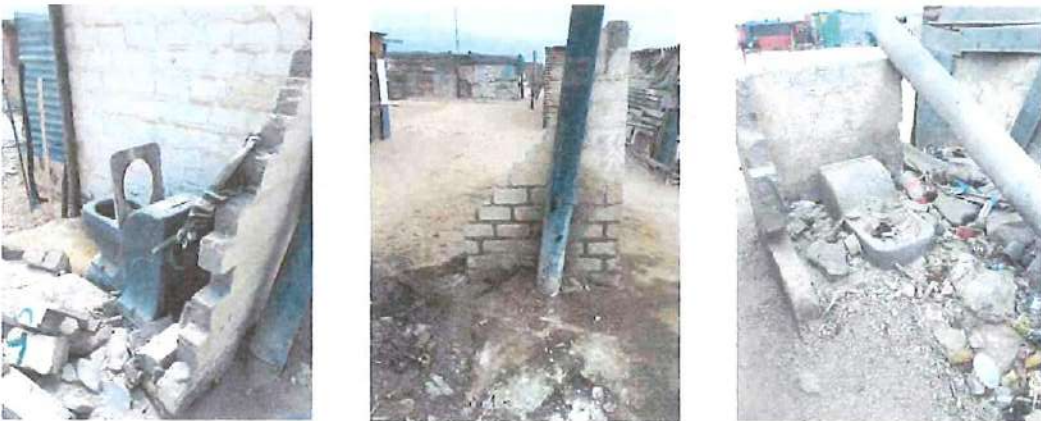
Figure 4. Destroyed structures of toilets in DRC Proper
