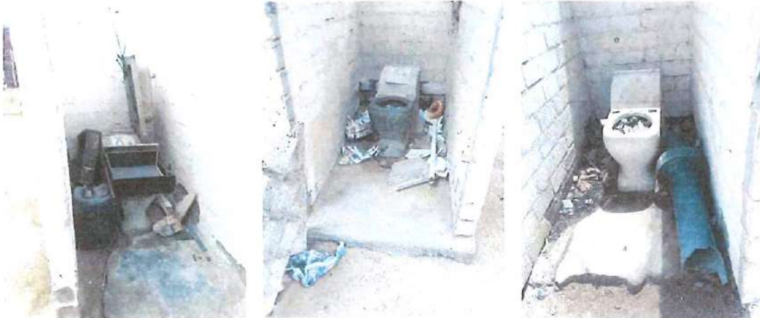
Figure 7. Toilets are abandoned and some used as storage facilities
