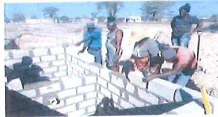
Women and men receiving toilet construction training in Zambezi informal settlement in Katima Mulilo
