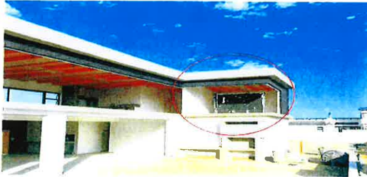
Figure 1: Unapproved enclosure on 1 st floor
