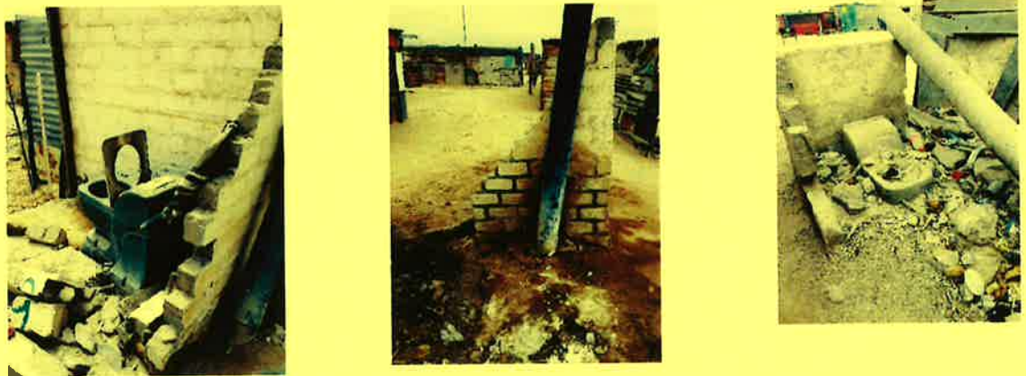
Figure 2: Destroyed structures of toilets in DRC Proper
